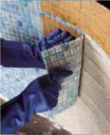
Glass mosaic 2x2 cm installation in a swimming pool with Adesilex P10 mixed with Isolastic diluted 1:1
